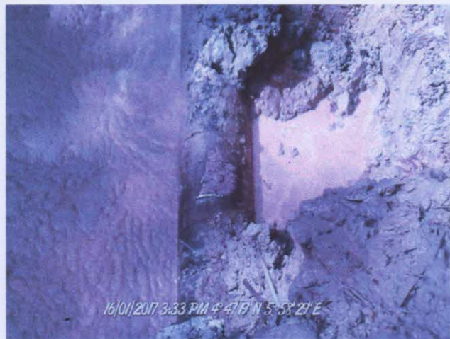
Figure 1: Cut-off Nipple on the pipeline.
